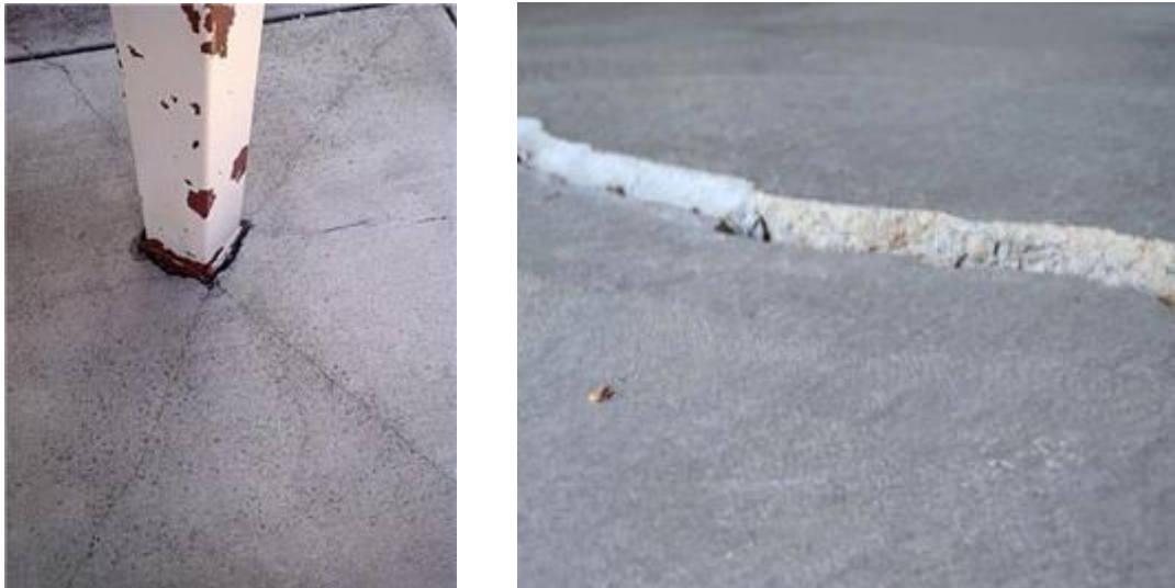
Figure 1.2: Plastic shrinkage cracks and settlement cracks
