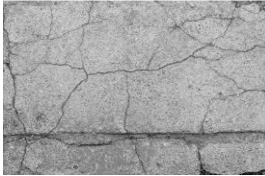
Figure 1.4: Cracks due to premature drying
