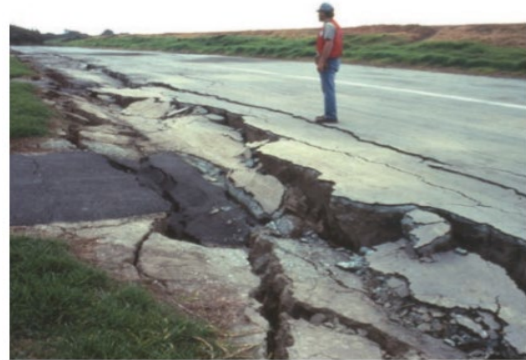
Figure 2.11 Lateral spread at in, California, USA, 1981
