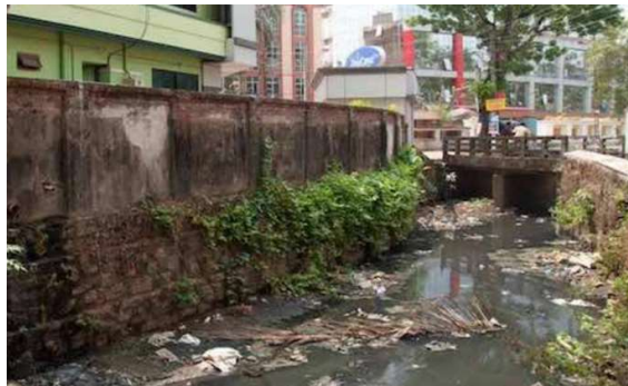
Fig 11. 3 Current drainage situation Guruvayur municipality Area which is badly effected
