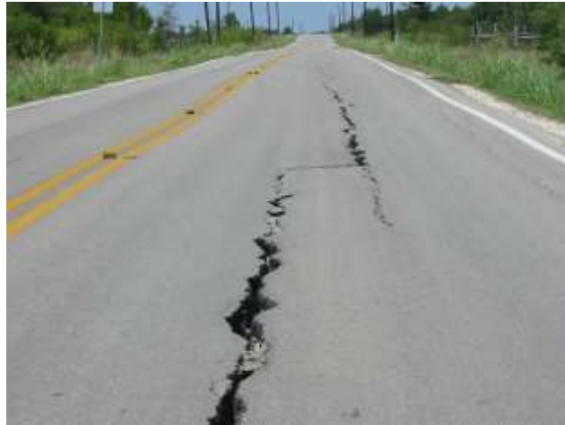
Fig. 1.1 Cracking in pavements
