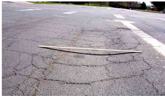
Fig. 1.2 Rutting in pavements
