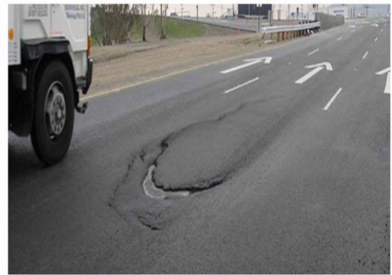
Fig. 1.2 Surface delamination (Source: Giri and Panda, 2018)
