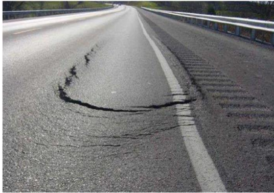
Fig. 1.1 Slippage cracking (Source: Buchanan and Woods, 2004)
