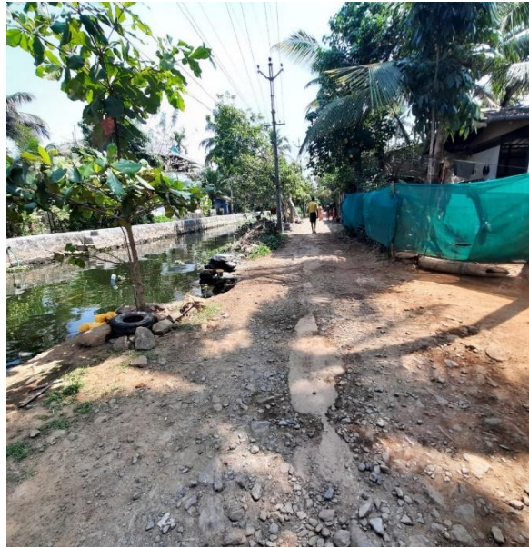
Figure 1.2 Condition of a rural road in Kainakary, Alappuzha
