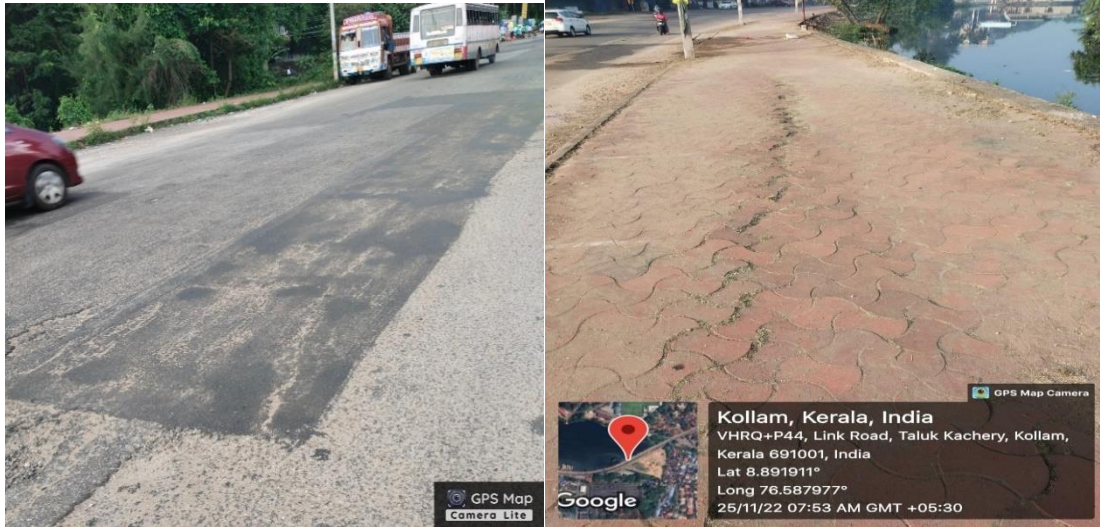
Fig. 1.1 Present condition of road section
