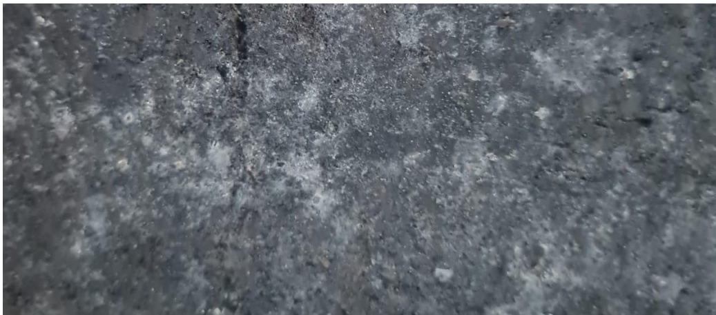
Figure 4.22- Formation of Efflorescence
