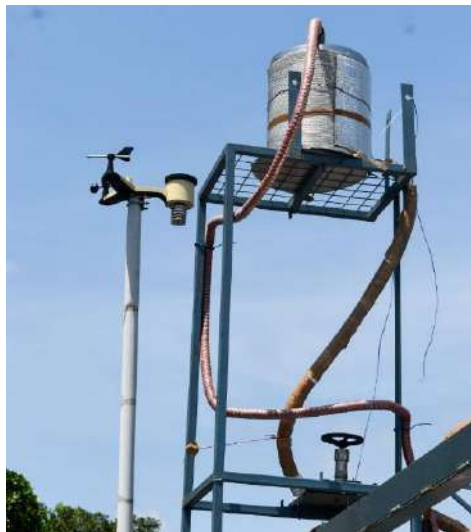
Fig. 5.21: HTF storage tank and weather station
