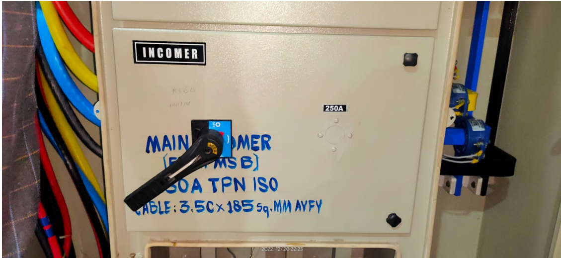
Fig. 5.3: UPS incomer where the hardware is installed
