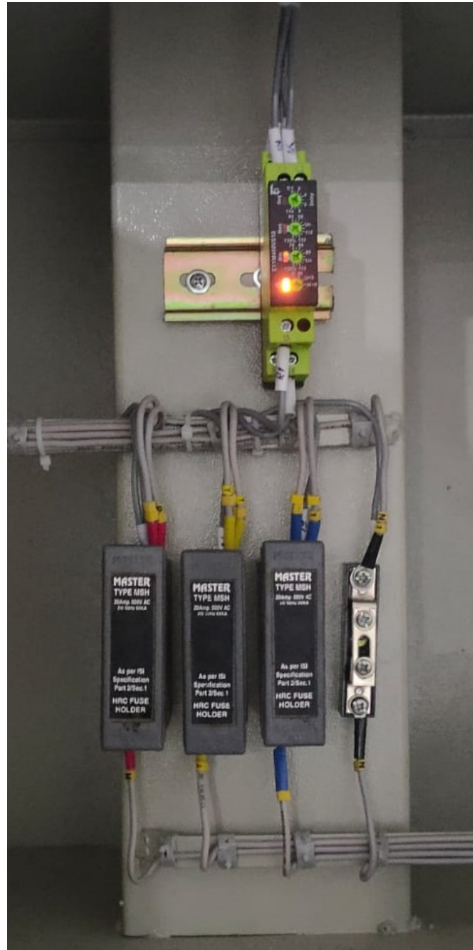
Fig. 5.5: Voltage monitoring relay connected to the line
