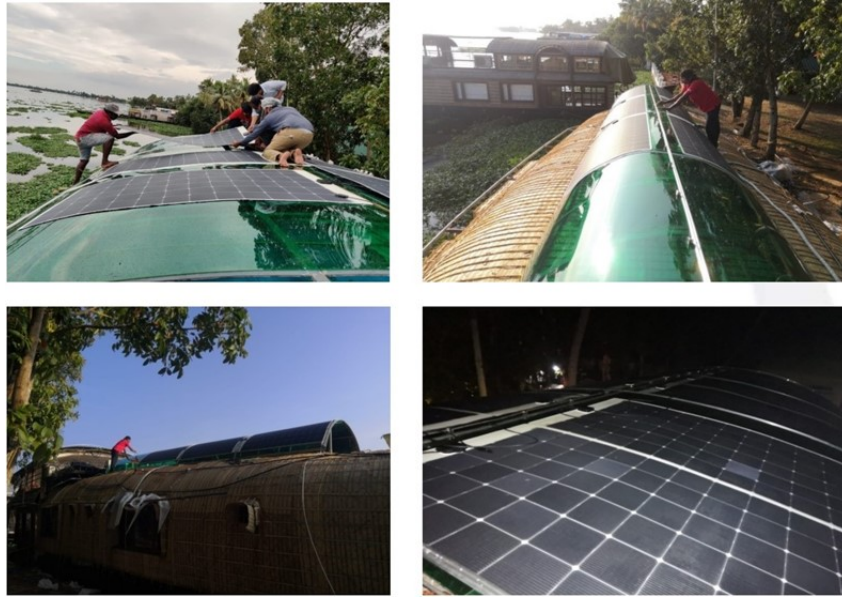
Fig. 8.2: Flexible solar panel placed on top of Houseboats for Cooking process
