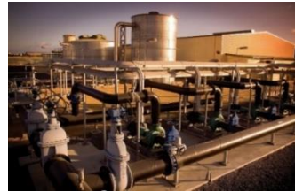
Figure 7.14. Water reclamation plant
