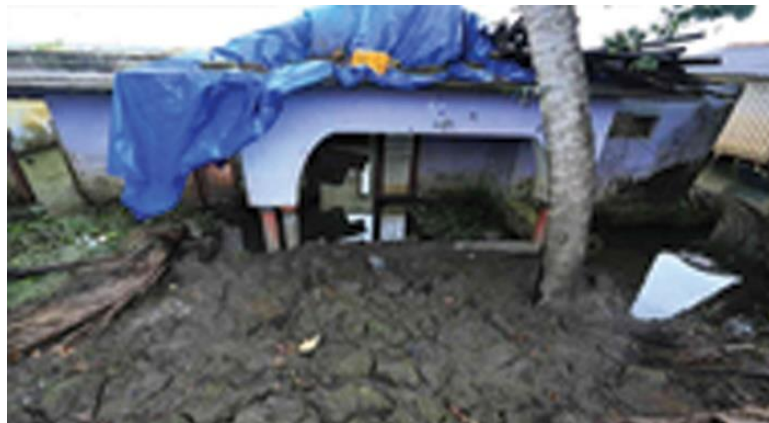
Figure 1:3: Abandon house in Kuttanad Source: Photos were collected from taluk office
