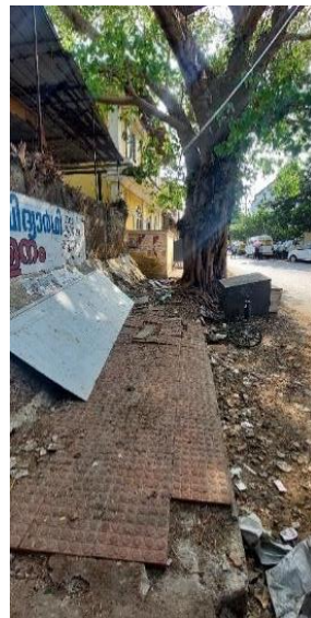
Figure 8. 8 Poor condition of footpaths.
