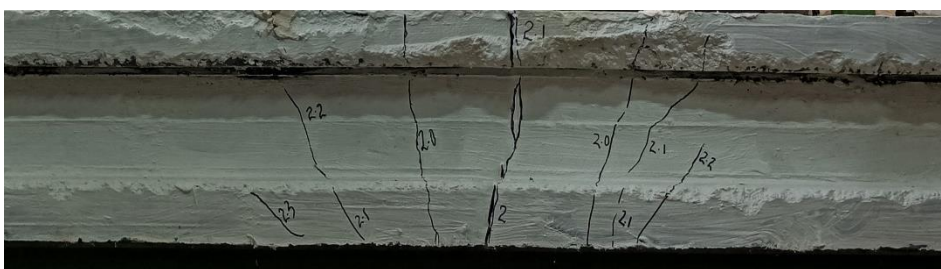
Figure 5.7 Crack pattern of SC Normal Mortar ferrocement I beam
