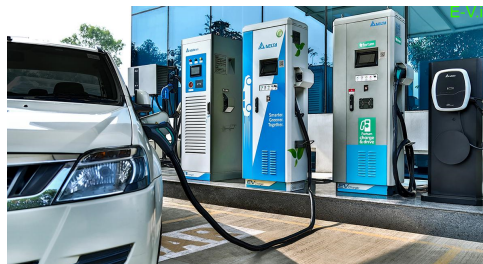
Figure 1.1: EV charging station
