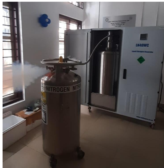
Fig 21. Liquid nitrogen production facility
